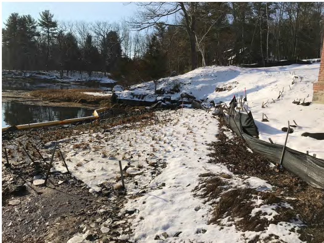
Fig 4: Toe of the slope and salt marsh restoration at the Eversource property/west side of the bay. Viewing south. (12-22-20)
