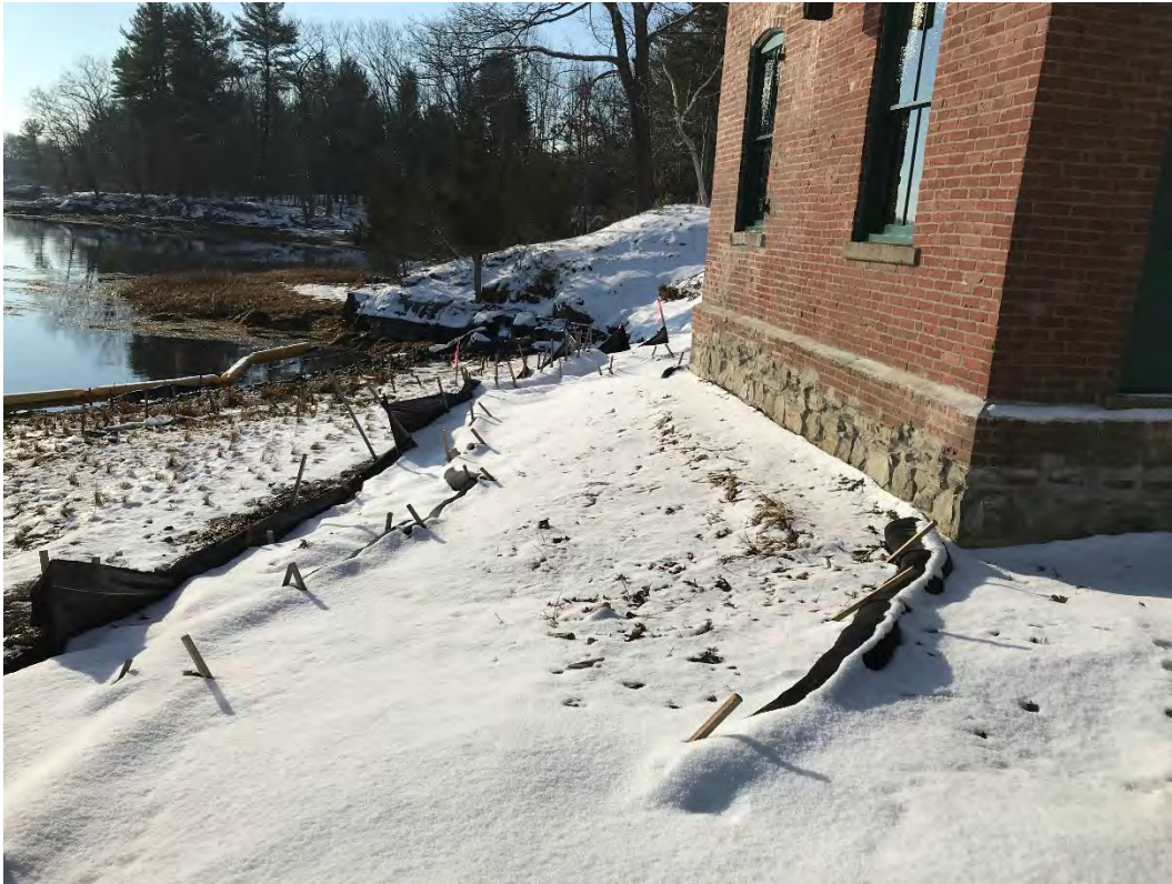
Fig 3: Slope between the cable house and salt marsh restoration at the Eversource property/west side of the bay. Viewing south. (12-22-20)
